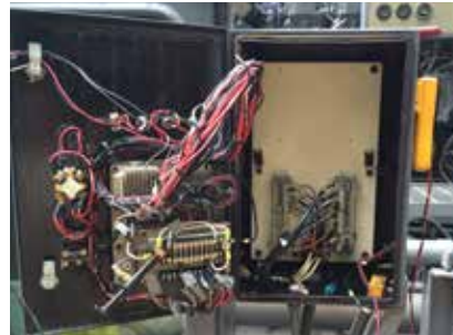
Wires have been disconnected; the ESCM is isolated and no longer a part of the system.
