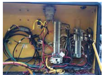
All wiring remains intact inside the engine-mounted panel. Future applications could replace the engine-to-ESCM panel's umbilical cable with a small 16-wire harness from Altronic.
