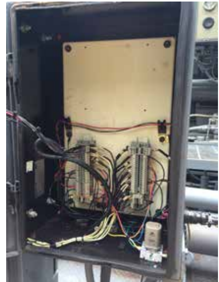
CAT items reused: terminal blocks, data port harness and cannon plug, umbilical cable from engine, and reset switch. New LED indicators were mounted in place of the OEM incandescent lights. Future systems will not reuse this housing. All components will be mounted inside a new Altronic control panel with new LED indicators, reset switch and terminal blocks. A small cannon plug with cable assembly (16 wires) will be used to connect the panel to the engine. A 10AMP relay replaced the OEM rotary switch.
