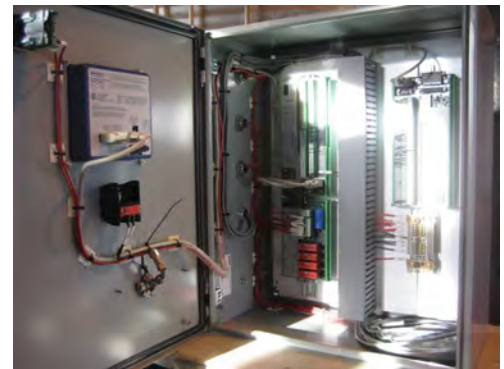
DE-3000 panel has room for expansion.
