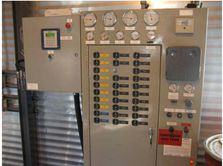
Existing pneumatic control panel with compact DE-3000 panel mounted on left side.
